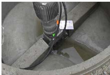
A 3-HYDRO-C Sewage Shredder with Immersible Motor at a Veterinary Clinic
